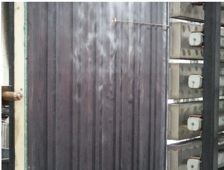
Photo No. 10 Bubbling of Exposed Surface
